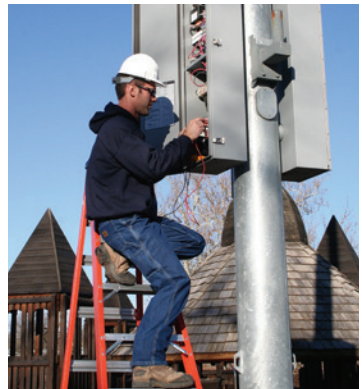
Having major electrical components accessible at ground level avoids hiring a $100/hour crane to replace a $10 fuse.
